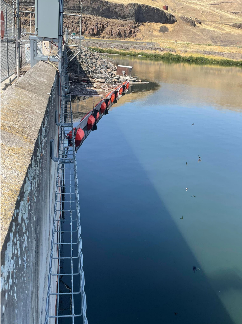
Image 3. Installed fish ladder debris barrier near the North shore adult ladder exit, Lower Monumental Dam.
